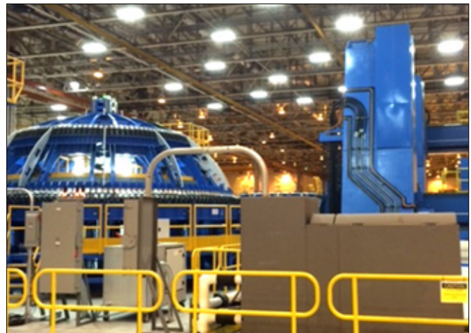
NASA's friction stir welder is used to create defect-free bonds for the new Space Launch System.
